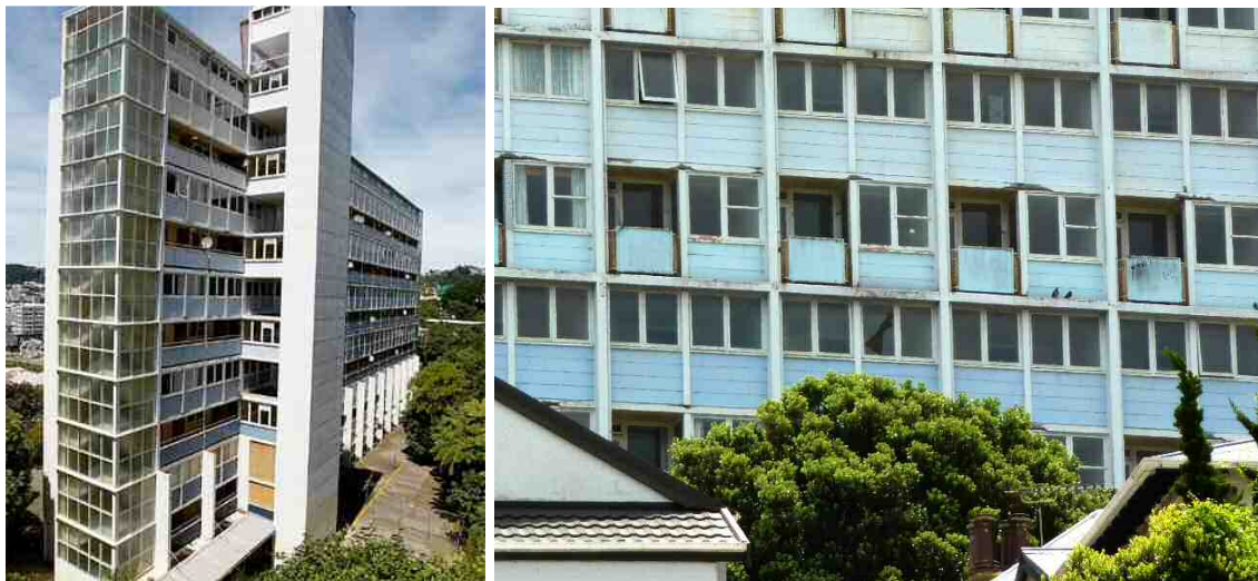
Gordon Wilson Flats: view of northern and western elevations | eastern elevation (in need of TLC)
